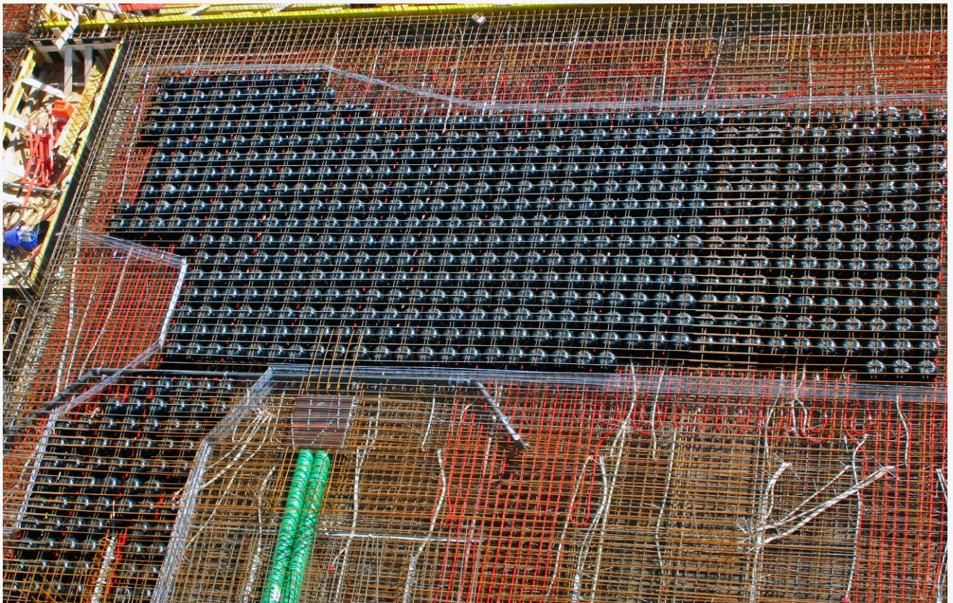
The most important thing was arranging seamless planning with everyone involved, to coordinate things like the positioning of the Cobiax modules and the piping for the concrete core activation well in advance. Source: Leonhard Weiss GmbH & Co.KG
