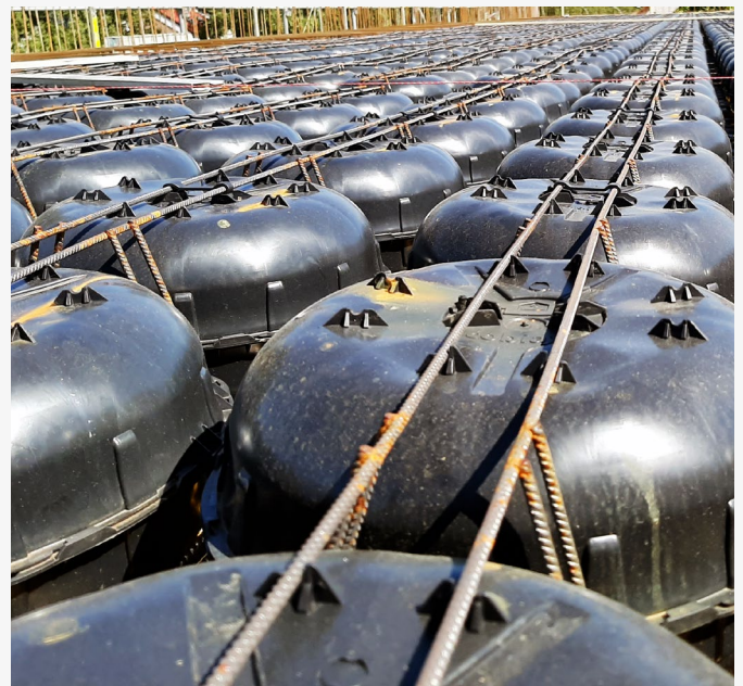
By using 34,398 Cobiax void formers, 1,210 tonnes of concrete have been saved in the new replacement building at the Ulm University of Applied Sciences. Source: Heinze Cobiax Deutschland GmbH
