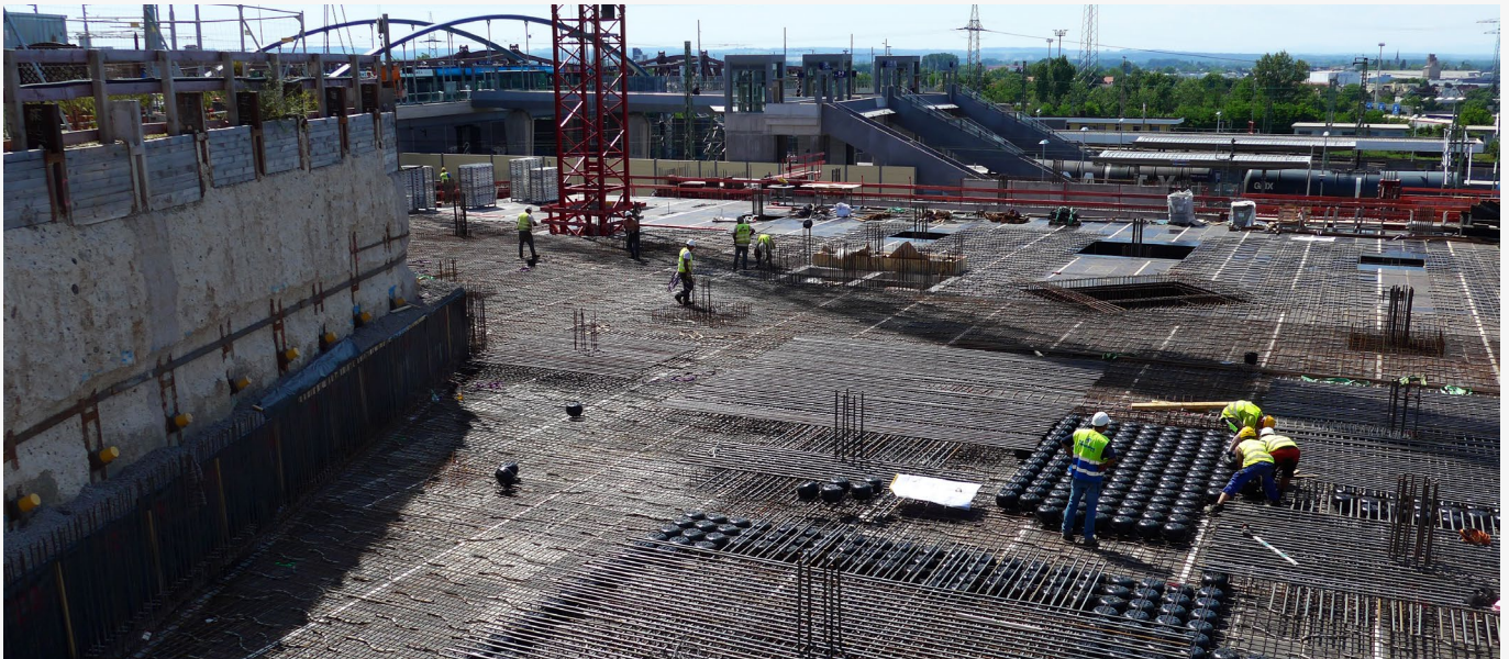
Around 108,000 void formers are used in precisely predefined, structurally non-critical areas, resulting in a total void former slab area of around 35,000 m 2 . Source: CEMAGG Weil am Rhein GmbH & Co. KG
