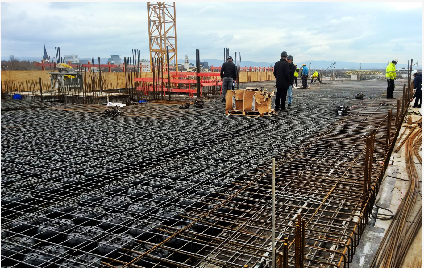
The modules are first set into a layer of concrete in order to avoid them bouncing around. The bond is created using the reinforcement steel elements of the void former modules, which at the same time serve to hold the individual void formers in place.
